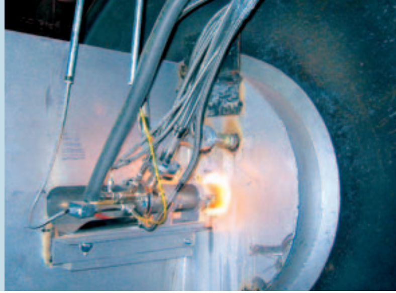
WASTOX® oxygen lances and oxyfuel burner in a double-pass furnace at Kuusakoski Oy, Finland.
