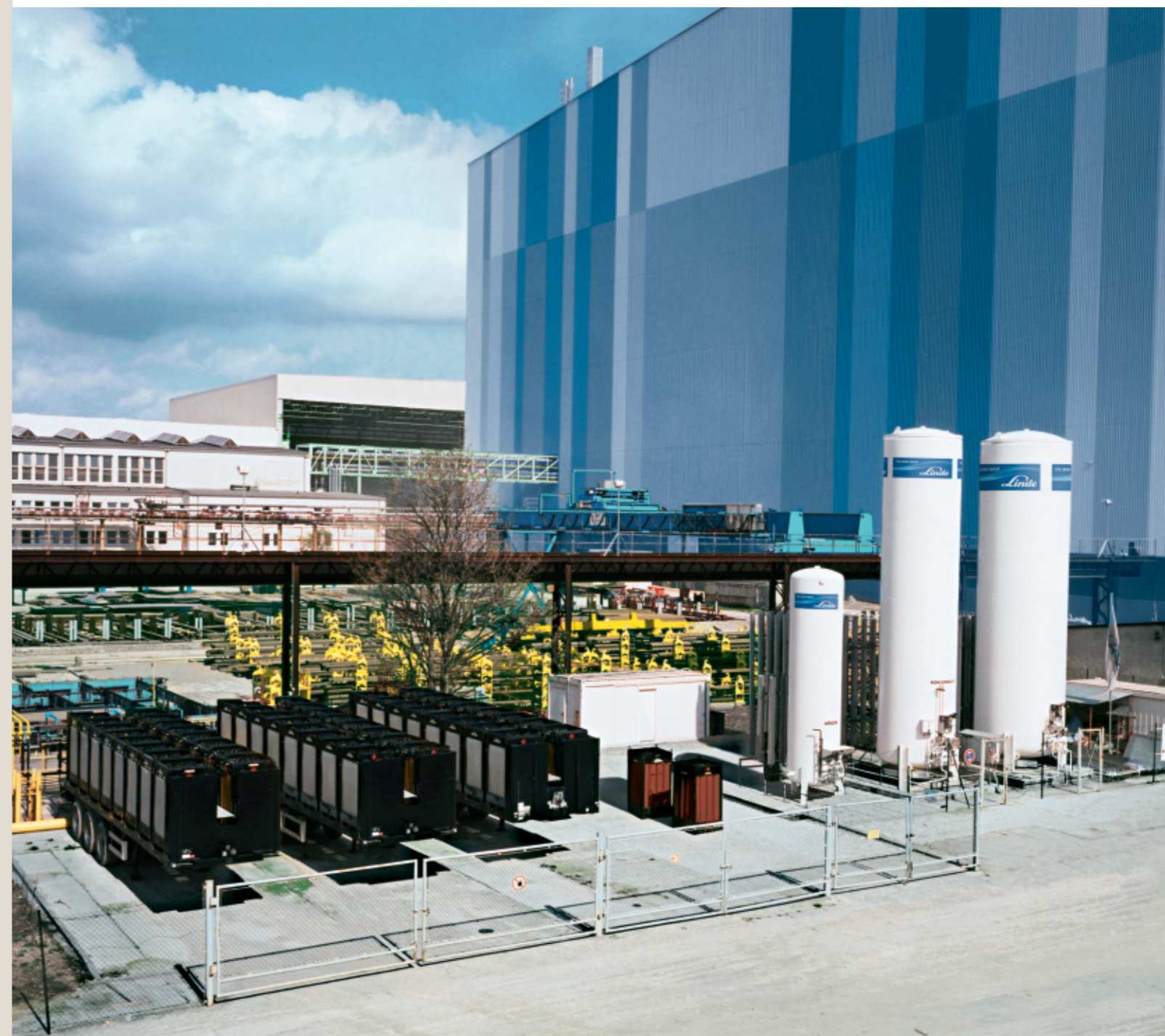
Gas supply point: three trailers for acetylene and liquid tanks for argon, carbon dioxide and oxygen.
