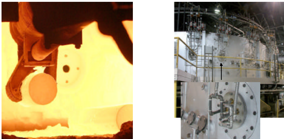
Figure 5. A look through the door and outside views of the REBOX ® installation in a rotary hearth furnace at ArcelorMittal Shelby.
