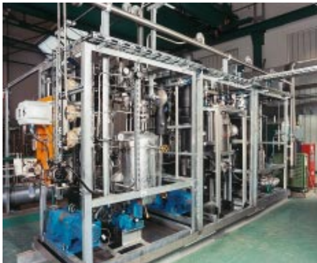
Figure 2: Test plant with peripherals
