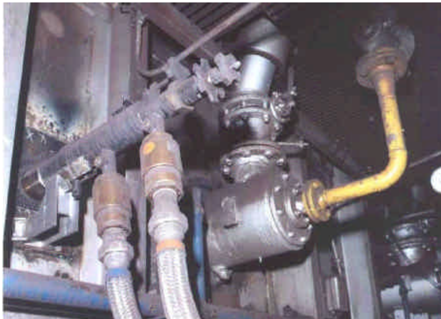
Figure 7: Oxyfuel burners are both compact and powerful. In this boosting application an additional 2 MW oxyfuel burner (left) are placed next to an existing 0.5 MW airfuel burner (right).
