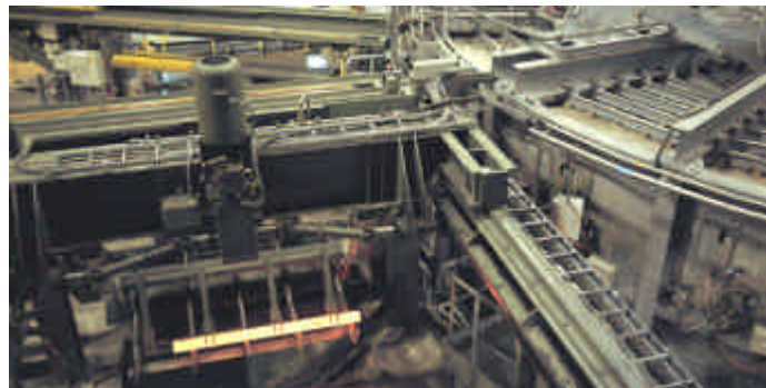
Figure 8: Rotary hearth furnace at Ovako in Hofors. Here billets, 170.000 tonnes/year, for tube rolling is heated with oxyfuel to a temperature of 1200°C prior to piercing.
