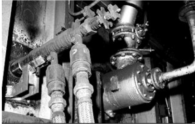
Fig 3. The 2 MW oxyfuel burner on the left in the photograph was installed for a boosting application next to the 0.5 MW airfuel burner in a pusher furnace.
