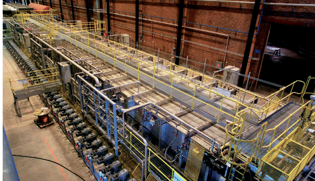
Roller hearth heating furnace with REBOX ® oxyfuel solution including ceramic oxyfuel burners and Linde control system.
