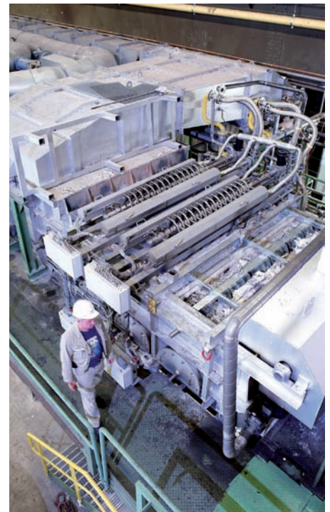
3 meter of the recuperative zone was used to fit the compact DFI oxyfuel unit.
