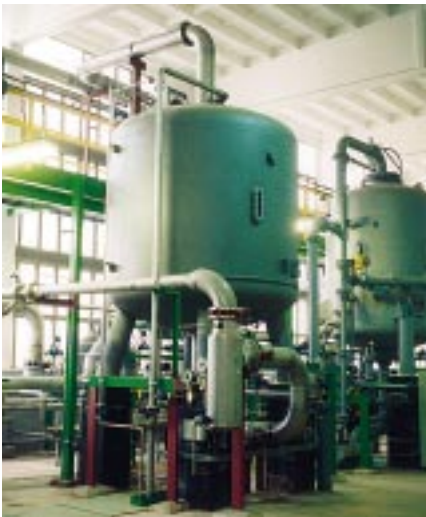
Catalytic reactor for deoxygenation of boiler feedwater
