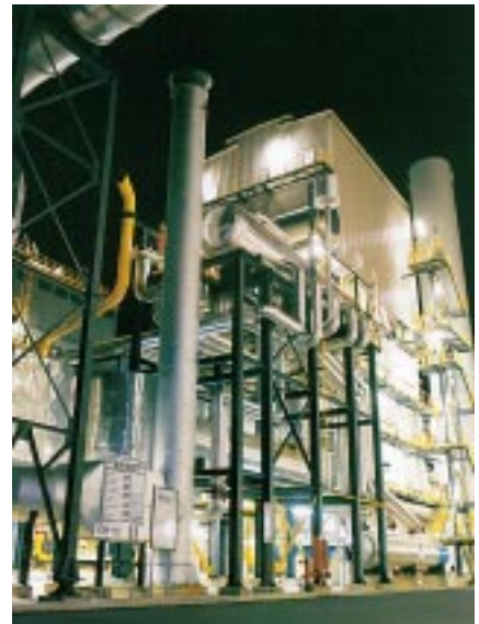
Steam reformer producing hydrogen in Milazzo, Sicily
