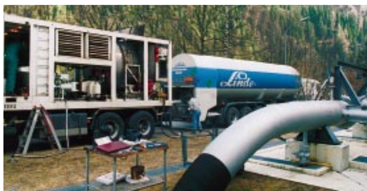
Pig trap and nitrogen feeding point in Rongellen, Switzerland
