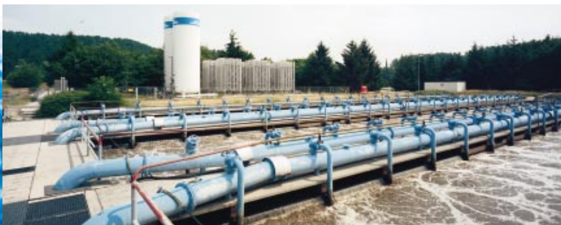
Oxygenation of wastewater using the SOLVOX®-B process
