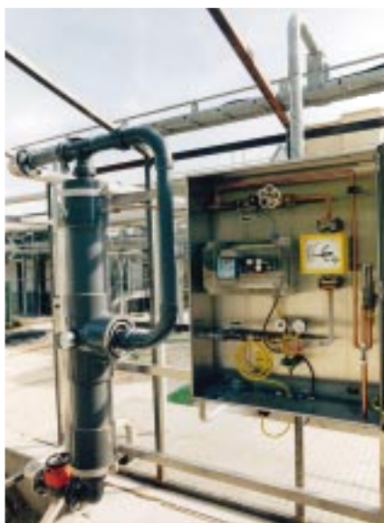
Neutralization with a SOLVOCARB® reactor in a chemical plant
